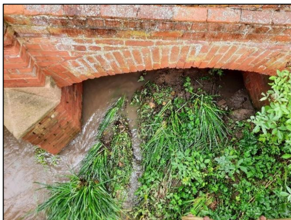
Photograph 11: Taken immediately after the event illustrating one of the twin arch bridges were partially obstructed (junction of Bridge Street and Mill Street)
