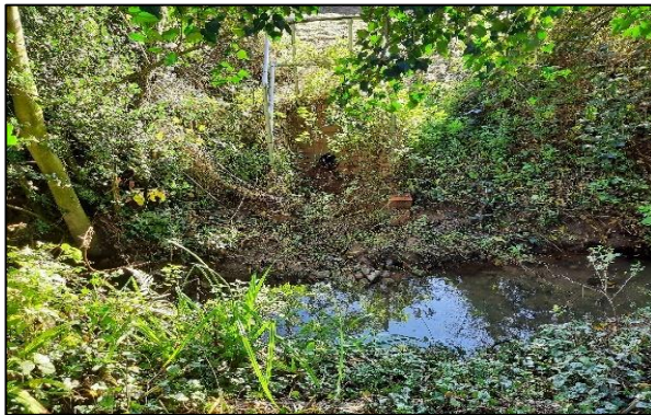
Photograph 8: Outfall into watercourse from estate. Located to the rear of 3 Heather Lane
