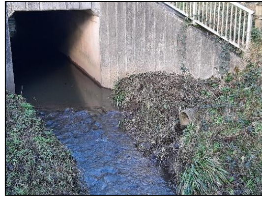
Photograph 2: Downstream of the A42 also showing a 300mm national highways outfall
