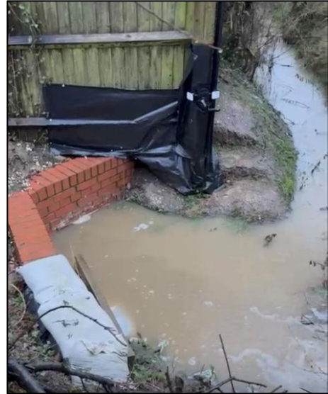
Photograph 4-2: 225mm dia culvert inlet submerged during wet weather – February 2026
