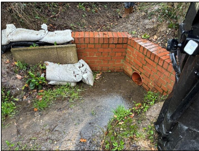
Photograph 4-1: 225mm dia culvert inlet during low flow conditions – December 2025
