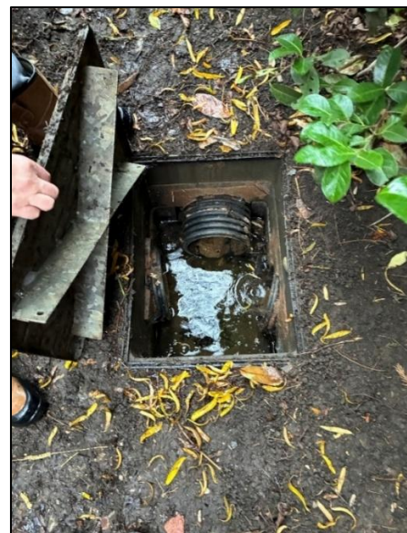
Photograph 4-4: Inspection chamber where high-level piped ditch ends before turning right into Fretter Close
