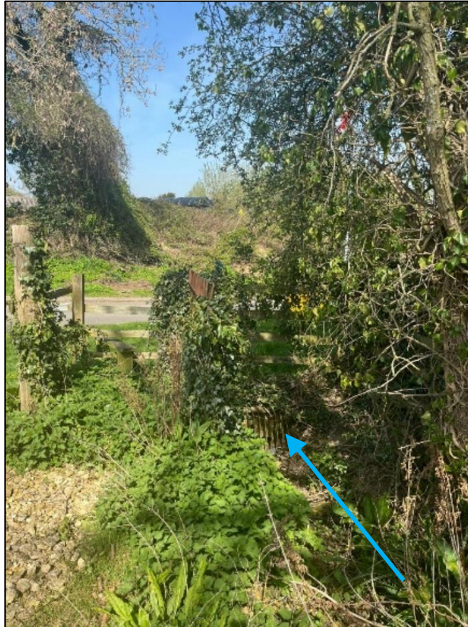
Photograph 6-7: Twin Culvert Inlet at downstream extent of Ordinary Watercourse 3 on the southern side of Rotherby Lane looking northwards
