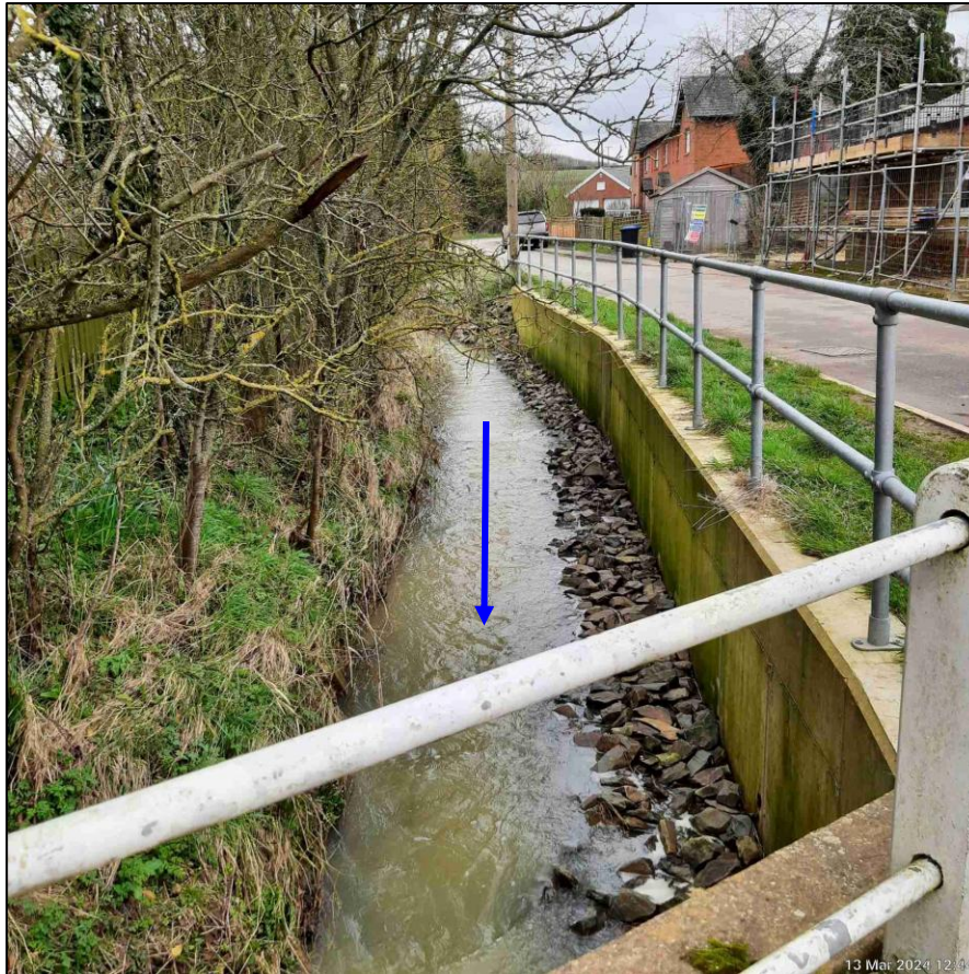
Photograph 7-6: Bank reinforcement upstream of Harbrough Road Bridge looking eastwards towards Cranoe Road
