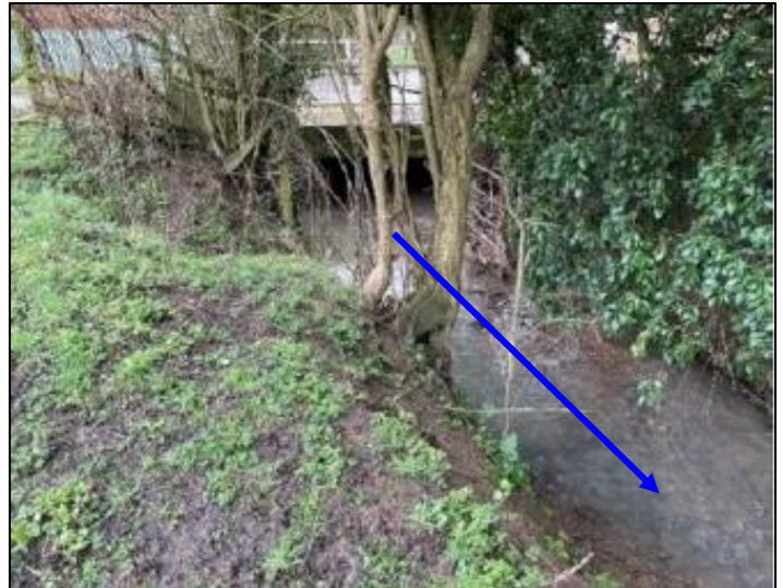
Photograph 7-2: Glooston Arm at the Harborough Road bridge culvert outlet looking upstream from Main Street3
