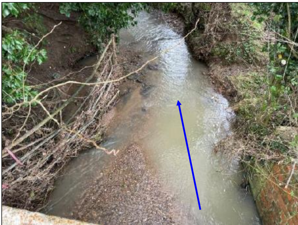
Photograph 7-7: Silt deposition within the Glooston Arm on outlet of the Harbrough Road Bridge culvert looking downstream following the flood event 3
