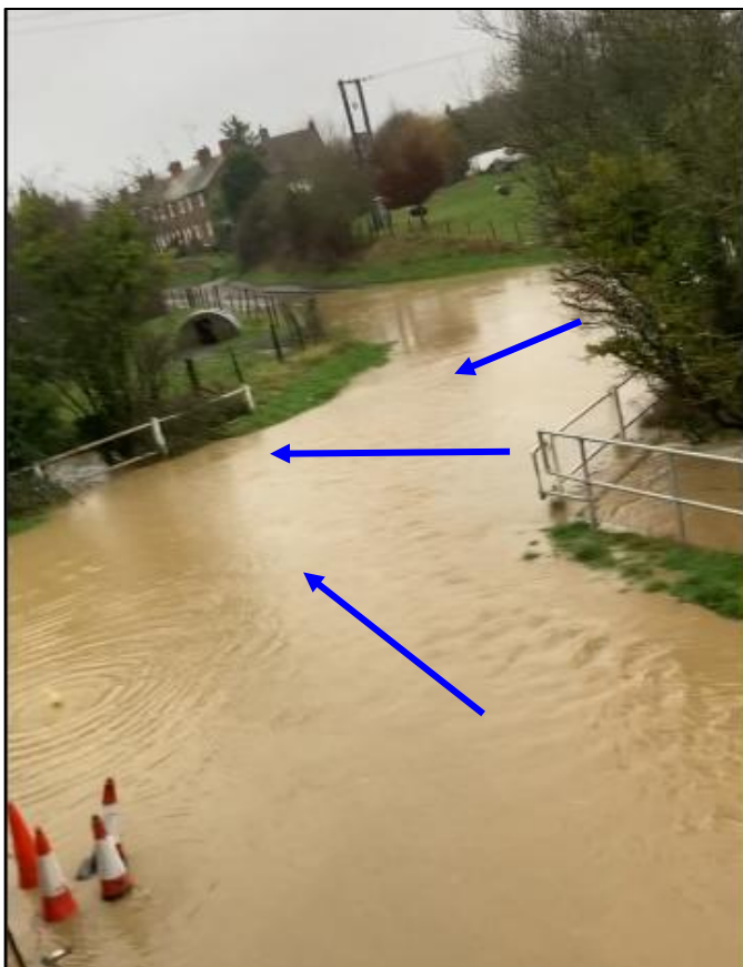
Photograph 7-4: View from Cranoe Road of Harborough Road bridge deck flooded looking downstream
