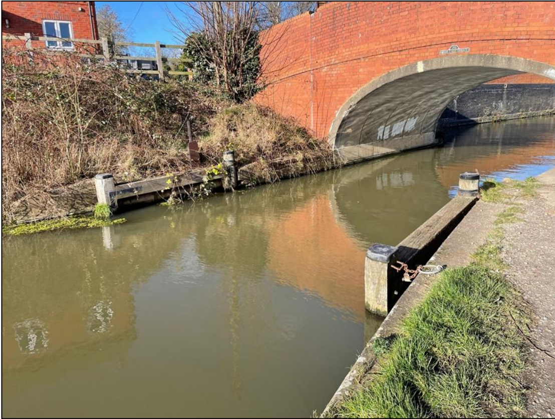
Photograph 8-4: Moor Lane Gates upstream of Moor Bridge on the Grand Union Canal 17
