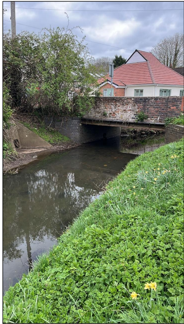
Photograph 17-5: Soar Brook in Sharnford looking downstream towards the upstream parapet wall of the Chapel Street bridge and STW CSO outfall
