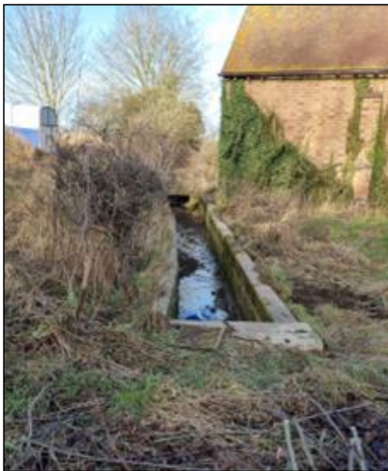
Photograph 20-1: Open watercourse in the field north of Main Street that flows into a culvert looking northwards
