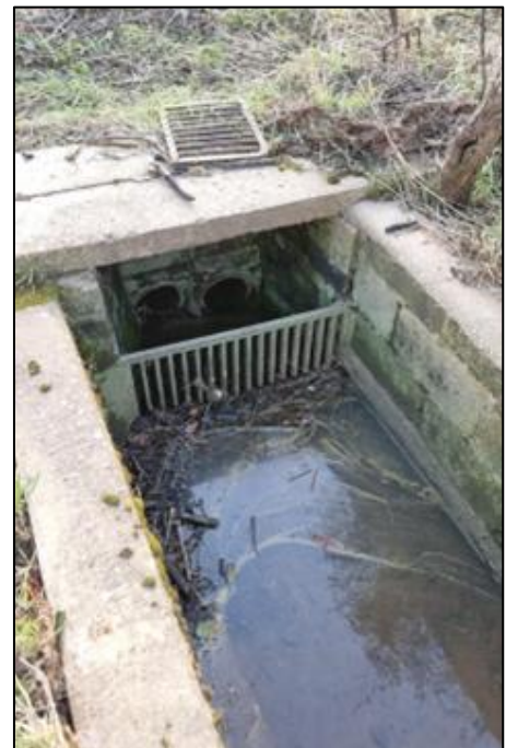
Photograph 20-2: Trash screen and culvert inlet at the field north of Main Street
