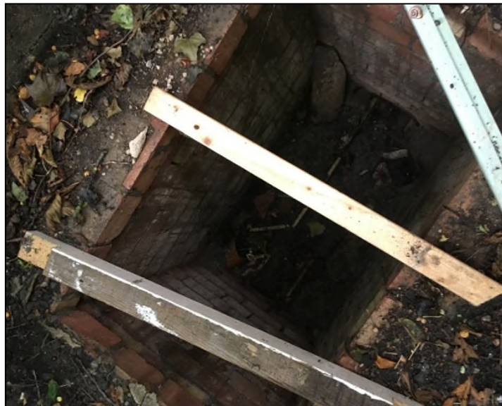
Photo 10: The inspection chamber which connects into the 100mm land drain and then Ordinary Watercourse 1.
