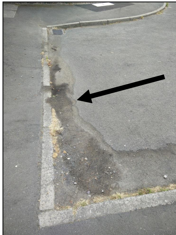
Photograph 1: Dropped kerb with sediment build up and gully positioning (top left) (arrow indicates direction of flow)
