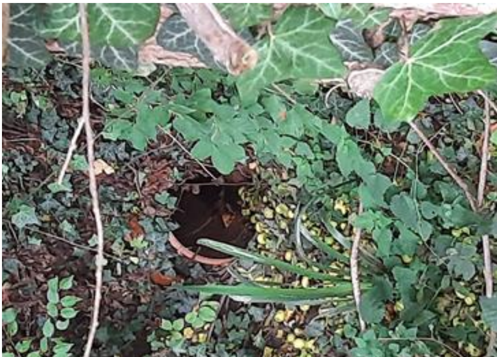
Photo 3: 300m culvert opening without a formal headwall which runs through the development site, as seen in purple on Figure 1
